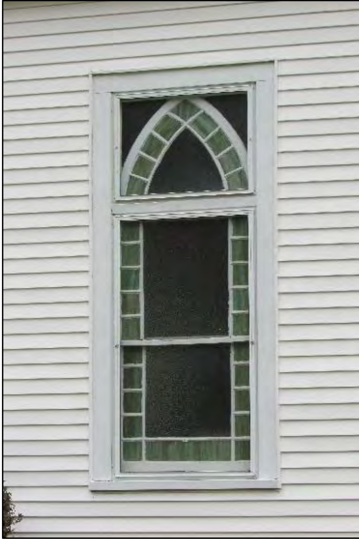
Figure 15. Hickory Baptist Church, detail of window on south elevation, looking north.
